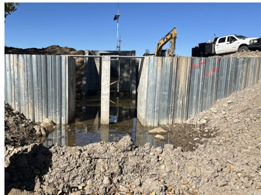
River water seeping into the kettle area
