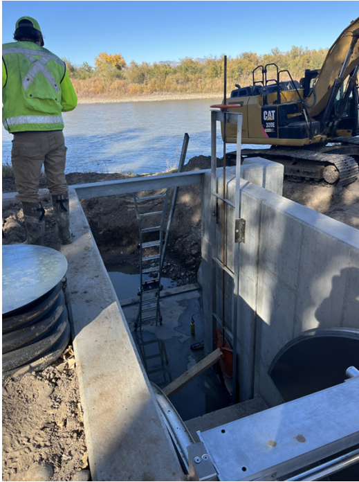
Preserve Project in the works: Entryway into the fish kettle from the Colorado River.
